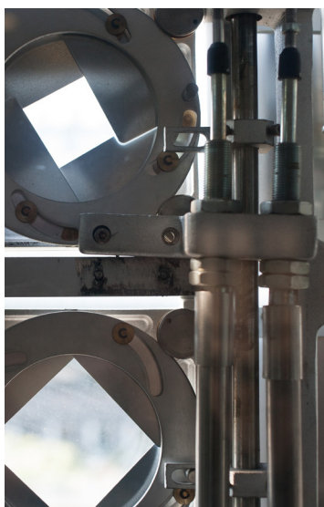
4.71 Institut du Monde Arabe. Structural failure of fastening bolts.
