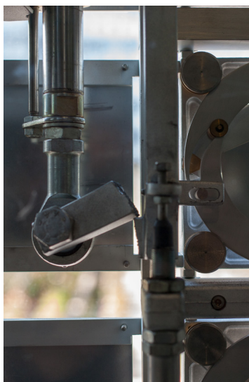
4.70 Institut du Monde Arabe. Structural failure of cast component.
