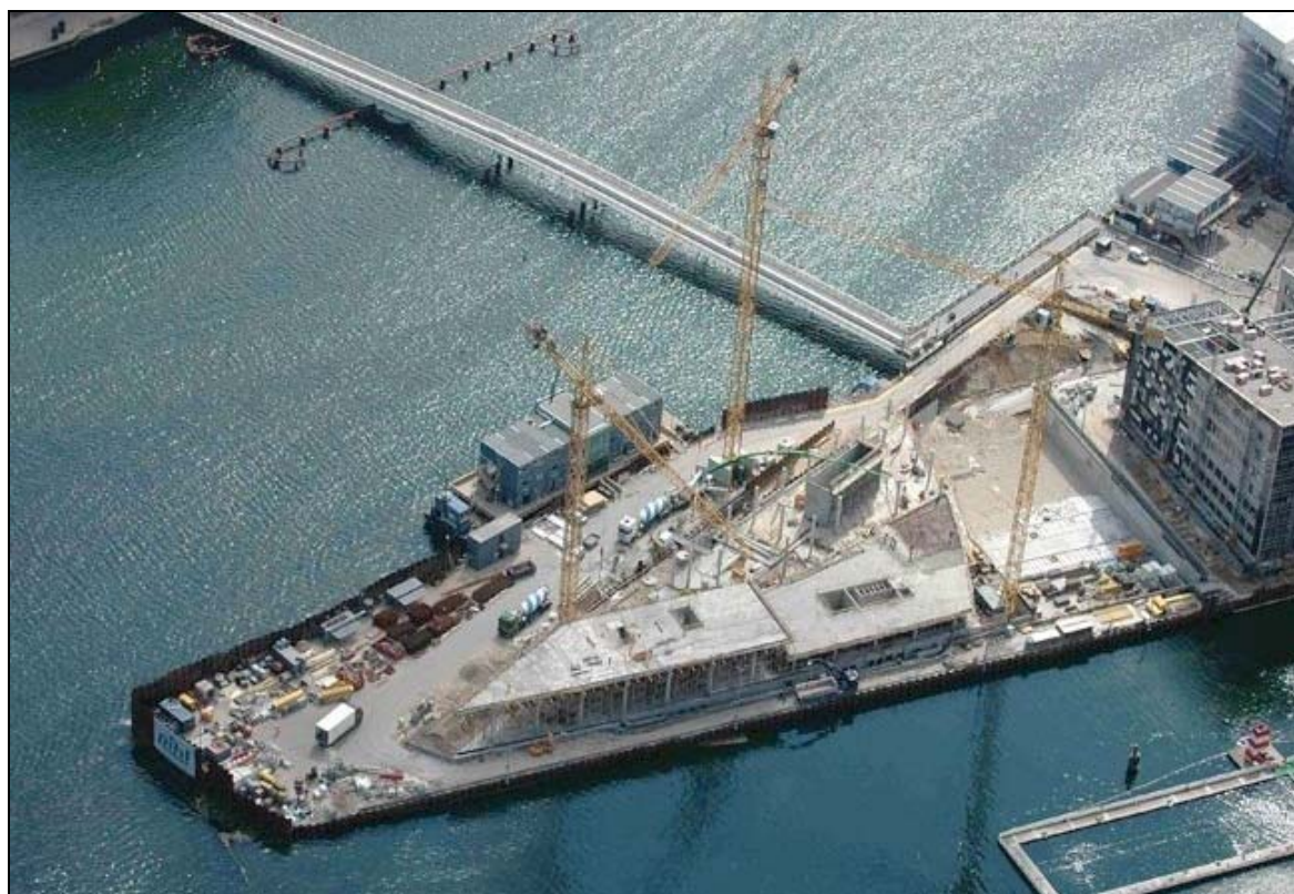
Figure 8: The superstructure in the initial phases of construction. Note the three kernels.
