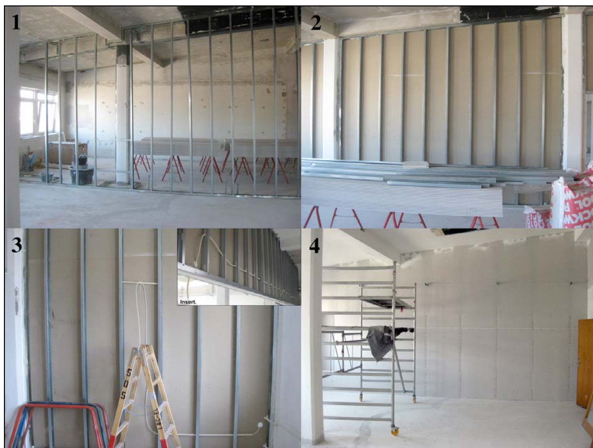
Figure 24: Interior wall in-the-making. The first and second frame shows the result of the carpenter's initial efforts. The third frame, including insert, shows the work of the electrician in progress. Finally, the fourth frame depicts the closed wall ready for painting.
