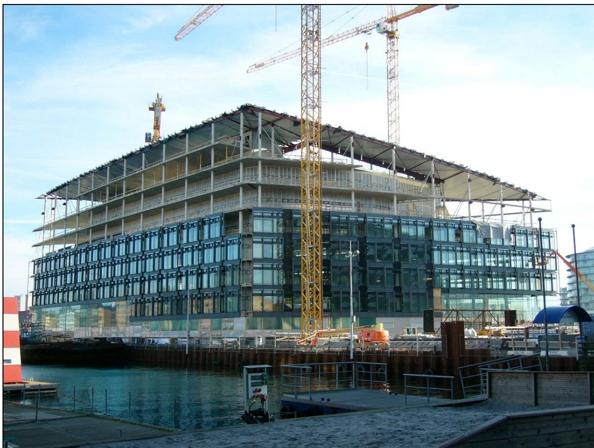
Figure 10: The domicile half-covered in façade panels and with some sections of the roof set in place.
